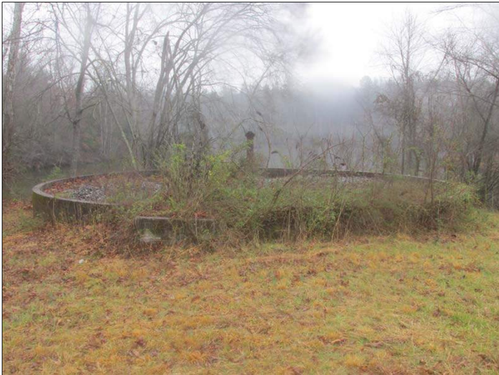
Photograph 8. Waste Water Facility at North End of Pearl Street, looking northwest toward Old Mill Pond
